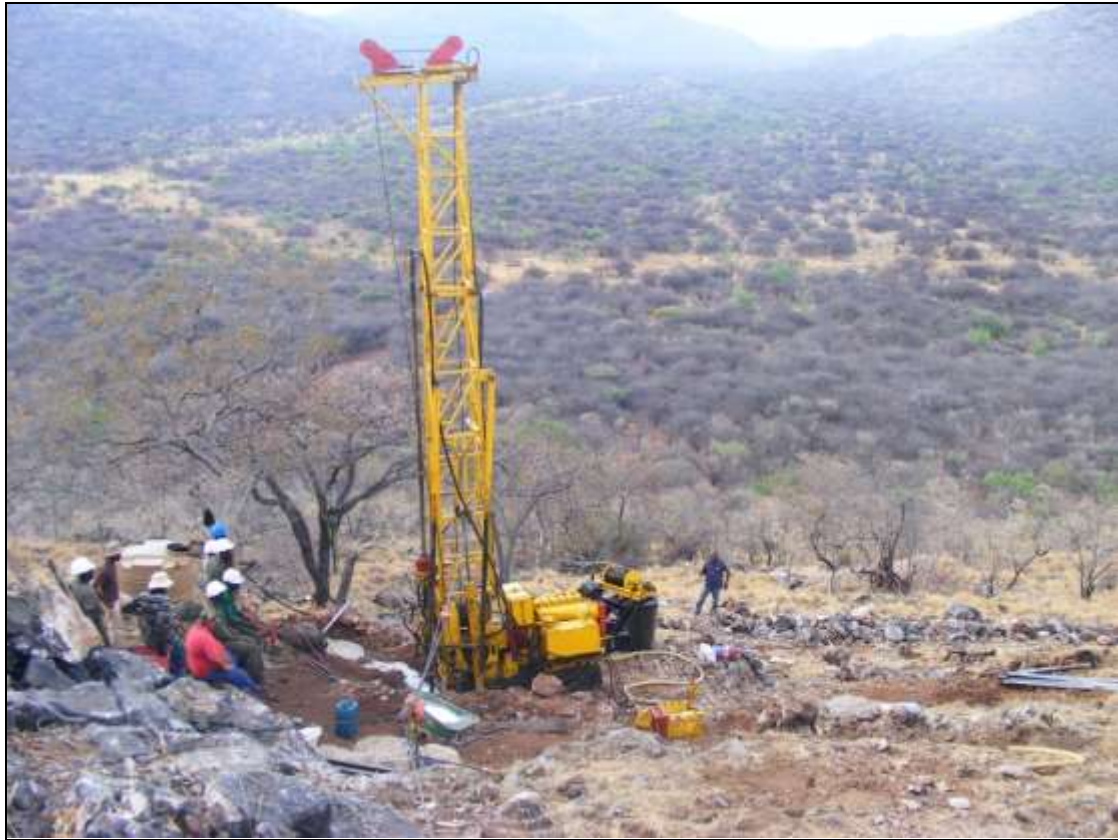
Figure 6 - The drill rig in position on the first drill pad at Kaskara.
