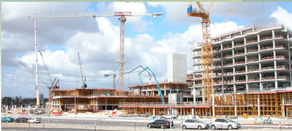
Construction of the $2 billion Fiona Stanley Hospital at Murdoch is proceeding on schedule. The hospital is expected to have a significant impact on the local residential property market well before it opens in 2014.
